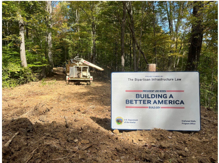
Figure 10: Gauley River National Recreation Area, BIL funded orphaned well site post plugging.
