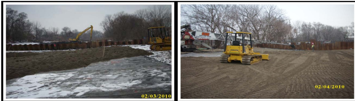
Placing sand cap and grading the north slope of Grand Calumet river bank (SulTRAC).
