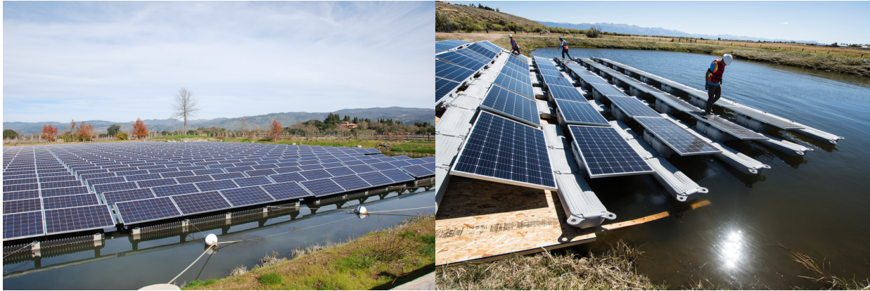
Figure 1 | Floatovoltaic installations can contribute to local- and regional-scale agricultural resource needs as demonstrated by this floatovoltaic system in Napa, California ( top , Photo: Far Niente Winery) and this floatovoltaic system under construction atop a water treatment facility in Walden, Colorado ( bottom , Photo: Dennis Schroeder, NREL).
