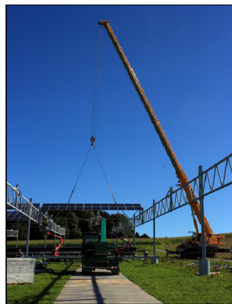
Fig. 5. (Right, source: farm community Heggelbach): Installation of APV power plant with mobile soil protection panels in August 2016.
