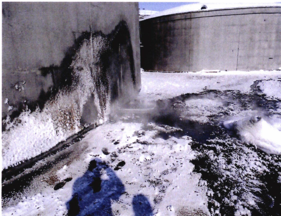
View north of piping vault where leak occurred
