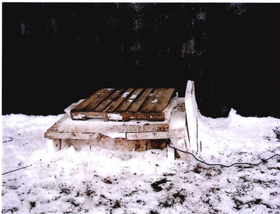
Insulation over piping well on digester w/out leak
