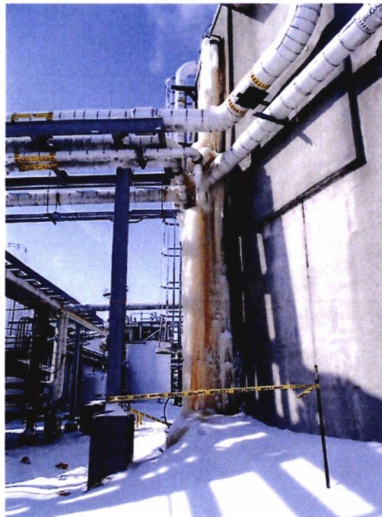
Spilling and leaking liquid from digester without leak
