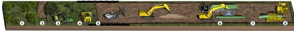
1. Survey and Staking 2. Access Road Development 3. Clearing* 4. Installation of Sedimentation and Erosion Controls 5. Grading 6. Stringing 7. Engineering Bends 8. Pipe Bending
