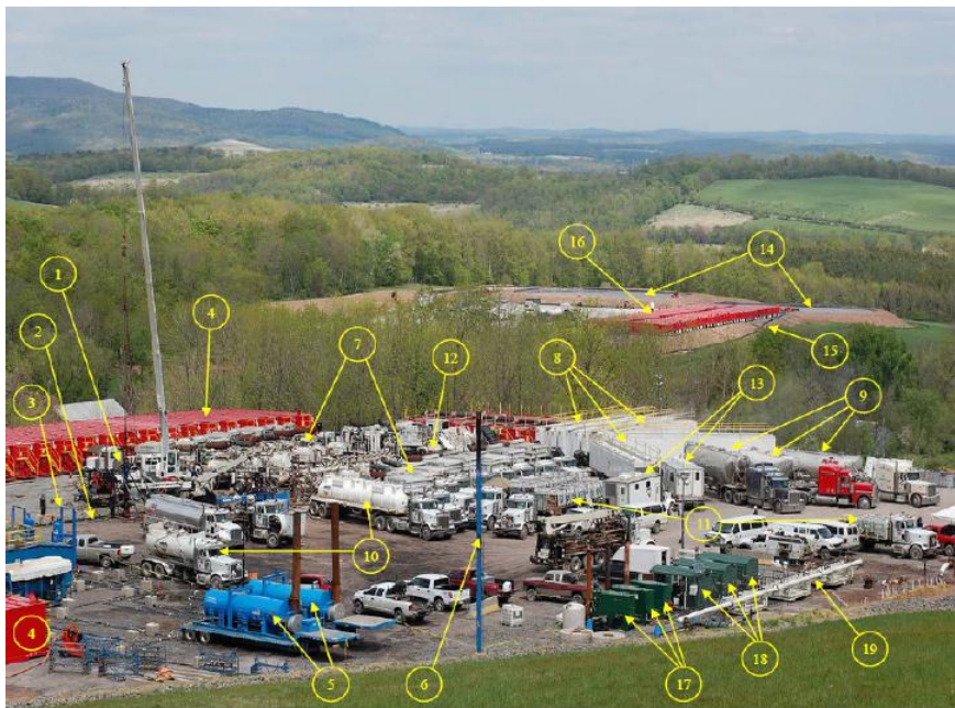
Figure 27: A shale gas well site during a single hydraulic fracturing operation (New York State, 2009) 14 [96]
