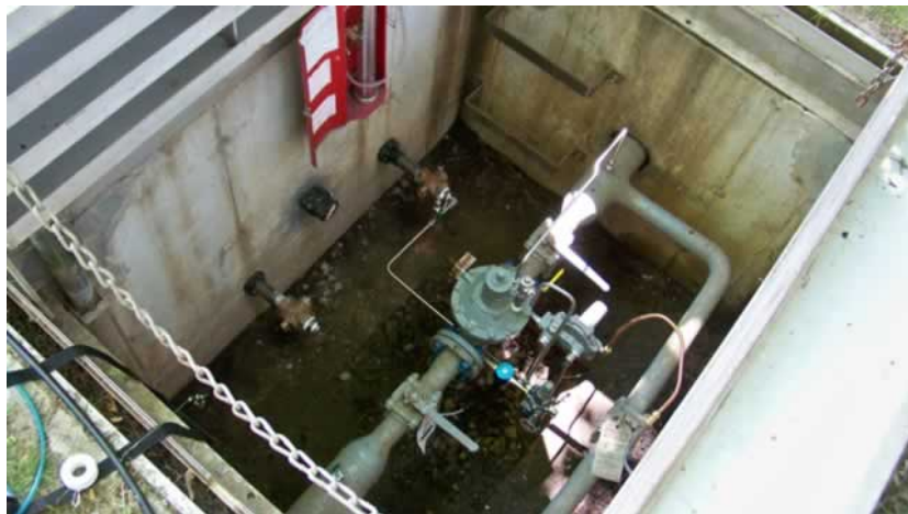
District Regulating Station –Vault Type
