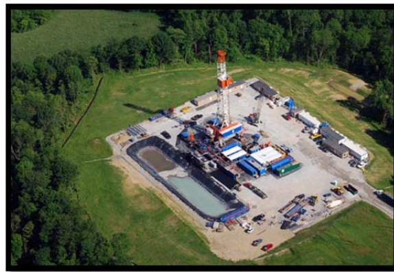
Figure 19: Example Well Pad in Pennsylvania (Photo courtesy of Robert M. Donnan, http://www.marcellus-shale.us/ )
