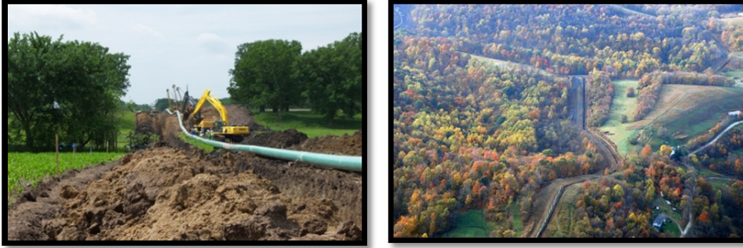
Figure 20: Example of Eastern U.S. Natural Gas Pipeline Construction (Photos courtesy of Robert M. Donnan, http://www.marcellus-shale.us/ )
