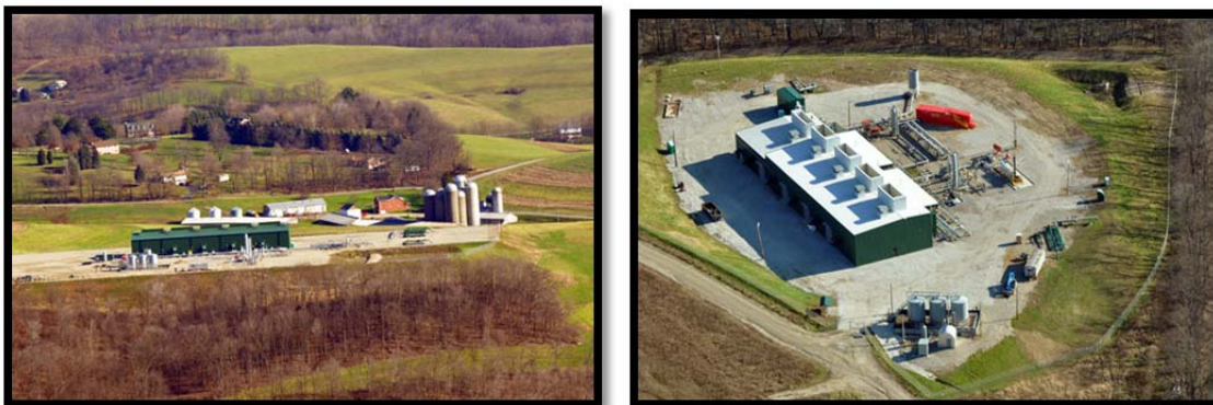
Figure 22: Examples of Natural Gas Compressor Stations (Photo courtesy of Robert M. Donnan, http://www.marcellus-shale.us/ )
