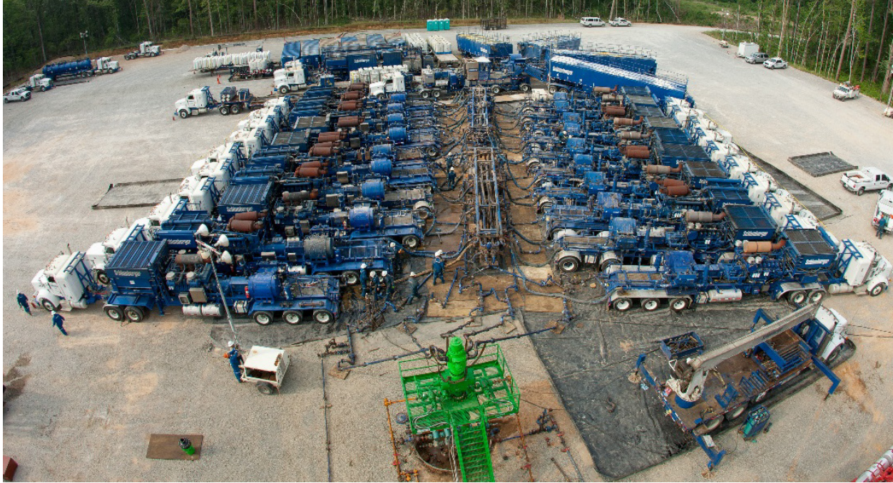
Figure 5-1. Representative hydraulic fracturing site showing equipment used on-site during the chemical mixing process.
