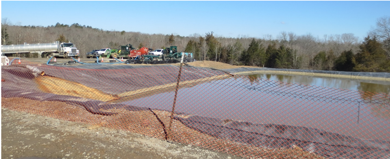
Figure 3-14. A pit on the site of a hydraulic fracturing operation in central Arkansas.
