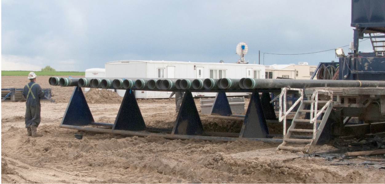
Figure 3-8. Sections of well casing ready for installation at a well site in Colorado.
