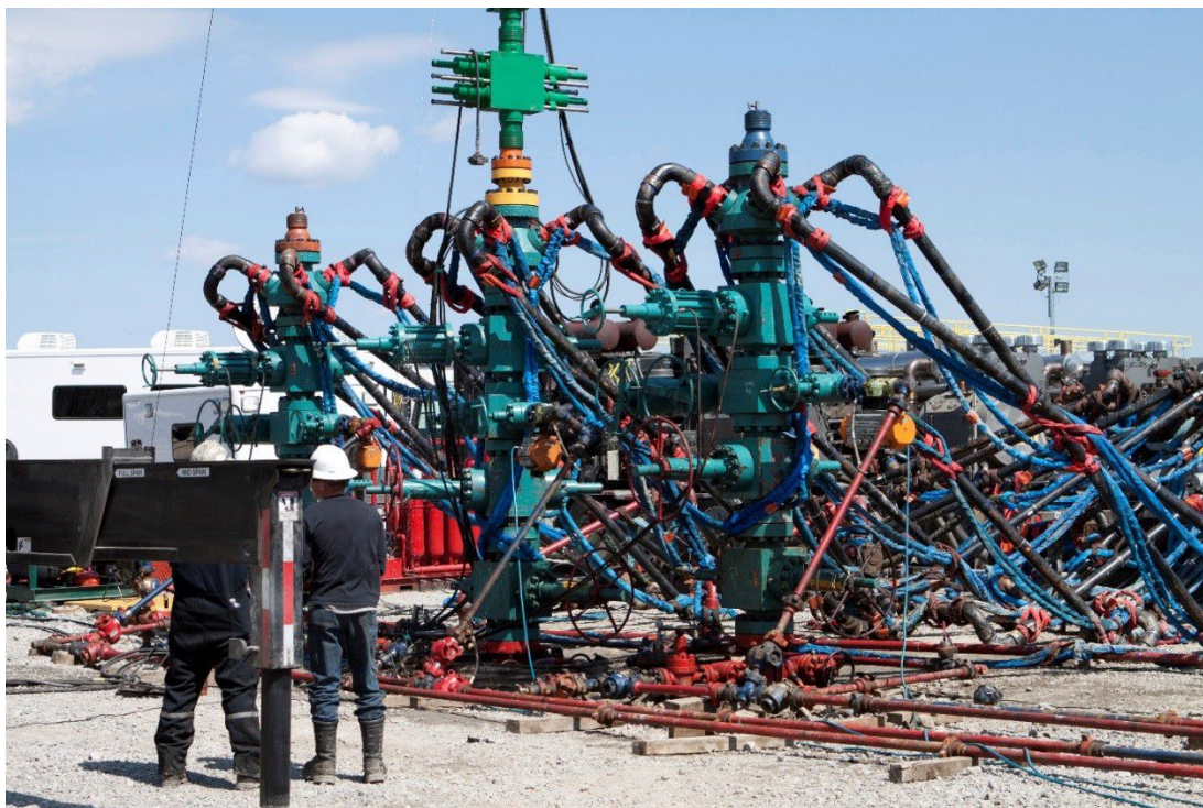
Figure 3-12. Three wellheads on a multi-well pad connected to the piping used for hydraulic fracturing injection.
