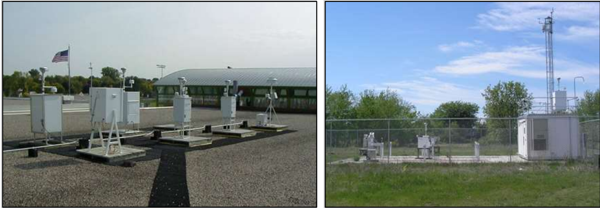
Example air monitoring sites: rooftop monitoring (left); ground-level monitoring including a shelter (right).
